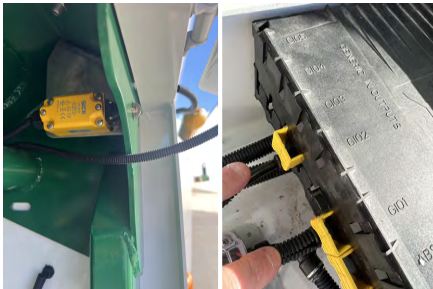
Figure 18: Left: Yellow Sick mechanical sensor is located on cabinet door. Right: RSS Module showing the wires connected to GIO3 and GIO1.
