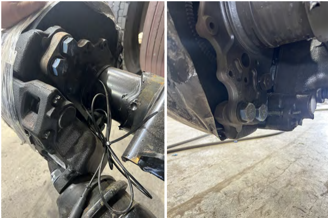
Figure 10: The Caliper assembly is secured with bolts shown in blue, these must be inspected quarterly to ensure correct torque. Failure to do so may result with loose caliper or even loss of caliper.
