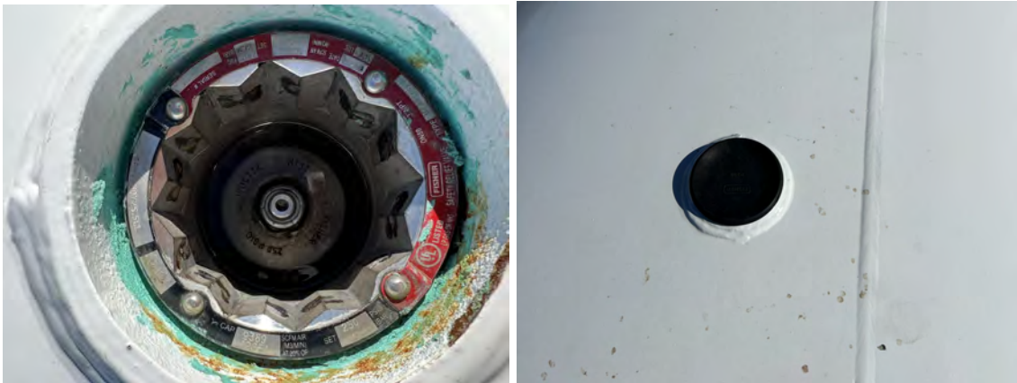
Figure 5: Left: Relief valve located on trailer top. Right: Relief valve with black plastic cap
