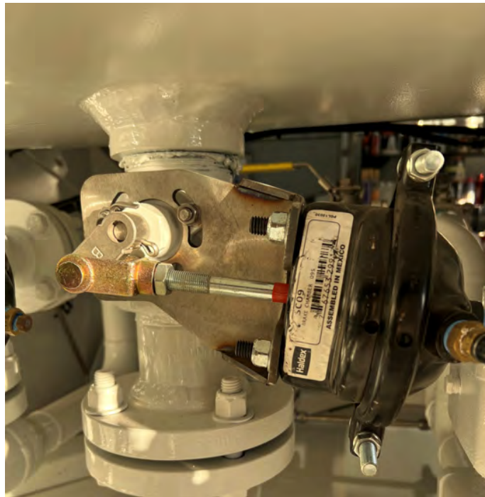
Figure 8: Shown actuator, black diaphragm piston pushes the rod which rotates internal valve clockwise via link.
